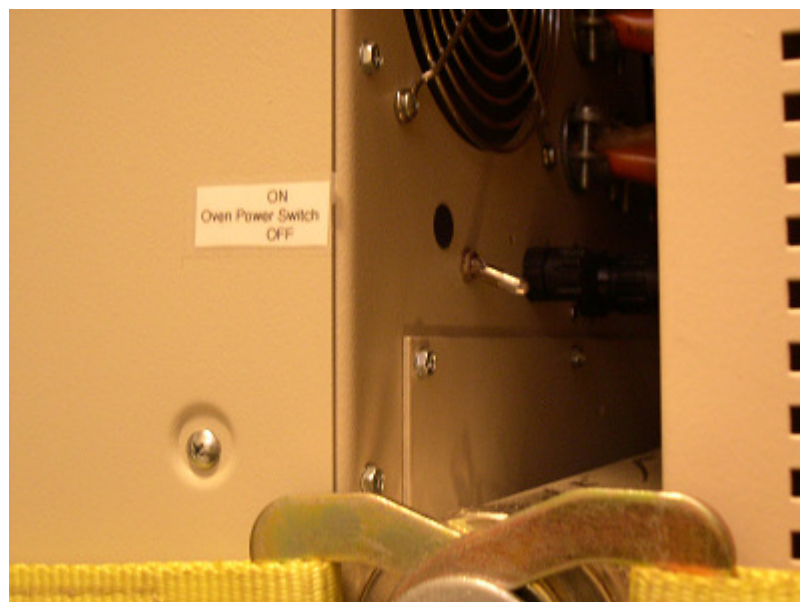
Foto 2: Interruptor del horno. (Oven Power Switch UPS Control Cabinet.)
