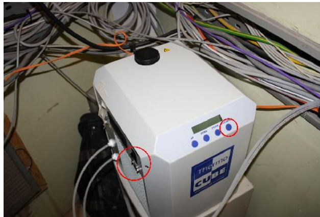
Figure 7. Cooler behind the rack of the telescope control PC.
